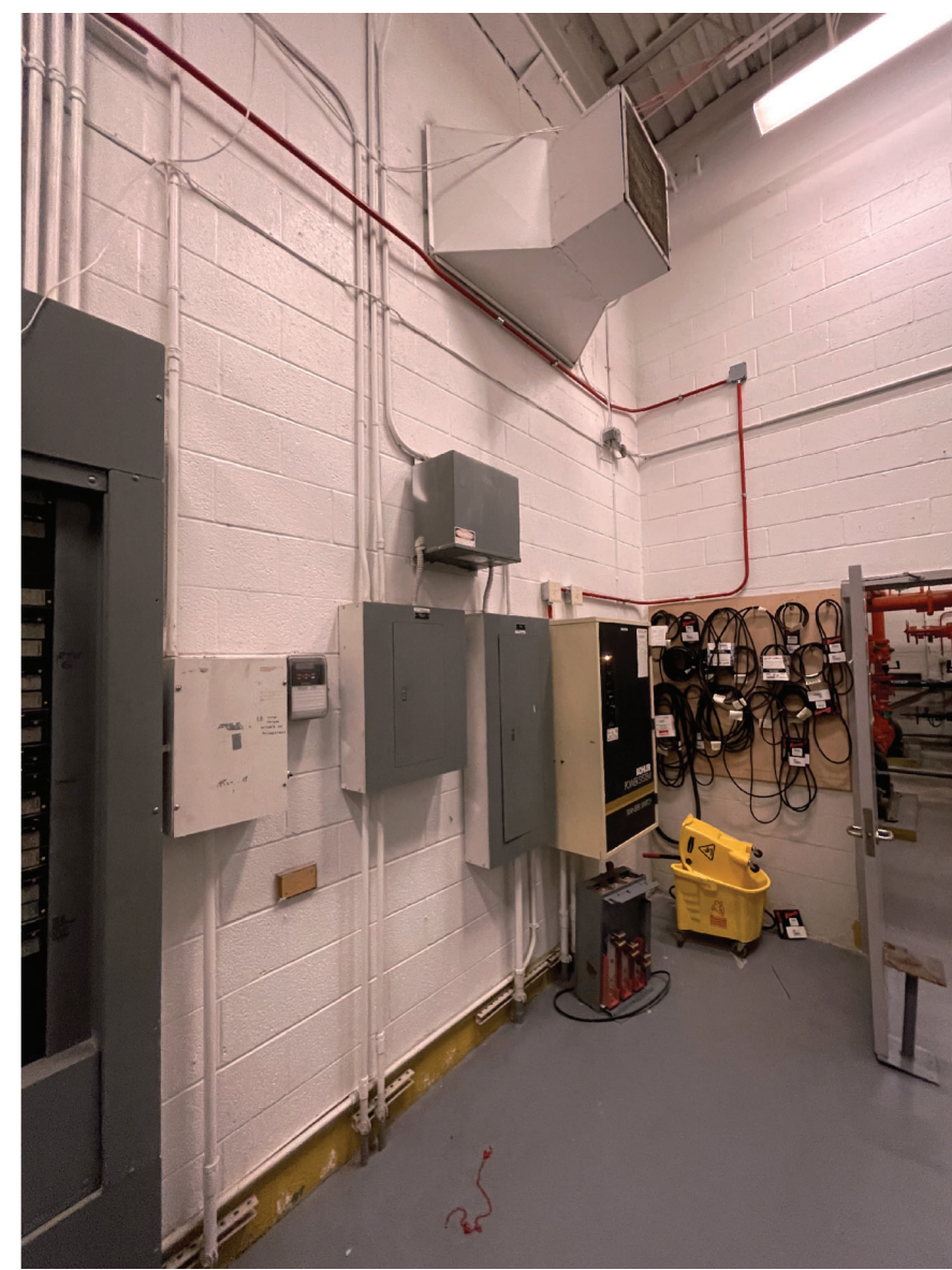
2 NEW EMERGENCY PANEL LOCATION
