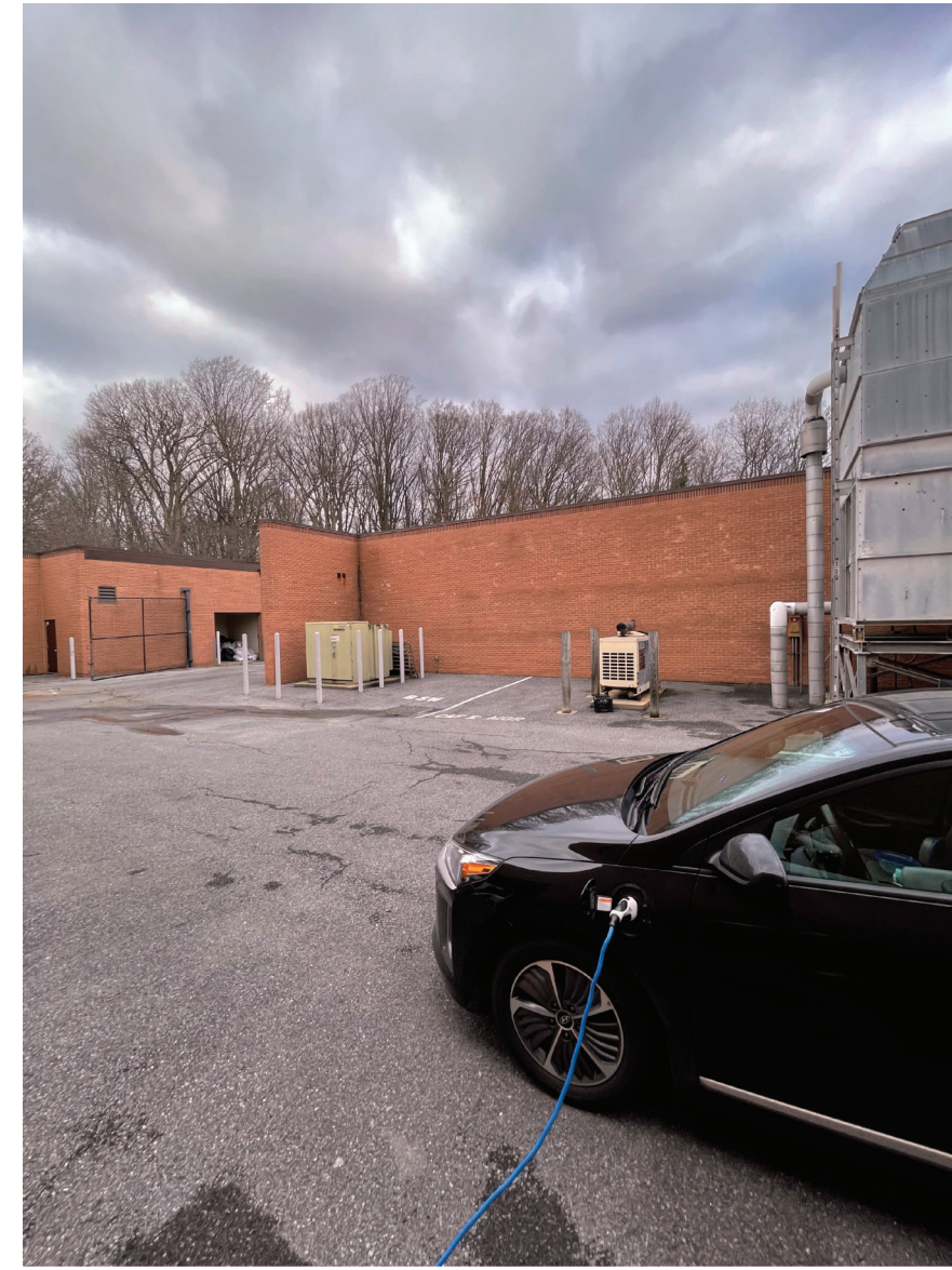
1 GENERATOR & UTILITY TRANSFORMER
